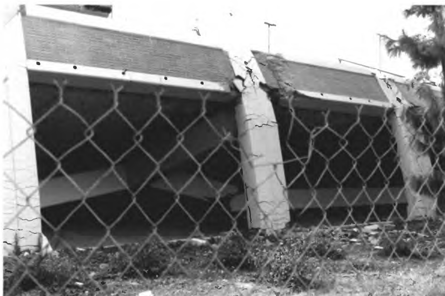
Figure 9. Collapsed parking structure at California State University at Northridge (listed under intensity IX).
