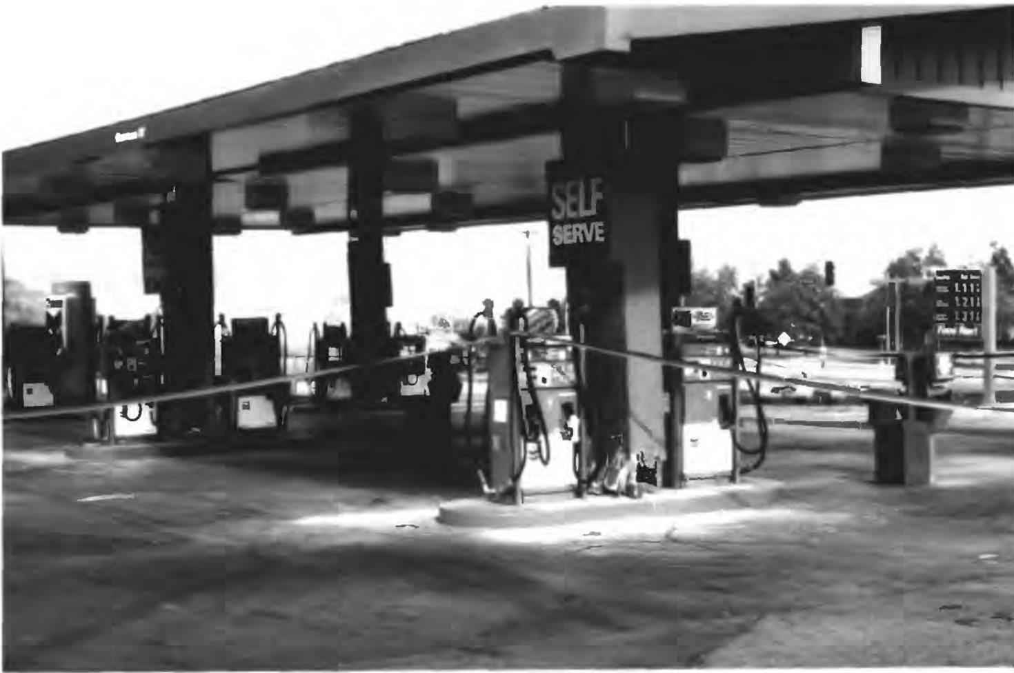
Figure 22. Damage to columns supporting a gas station canopy, near Stevenson Ranch (listed under intensity VIII).
