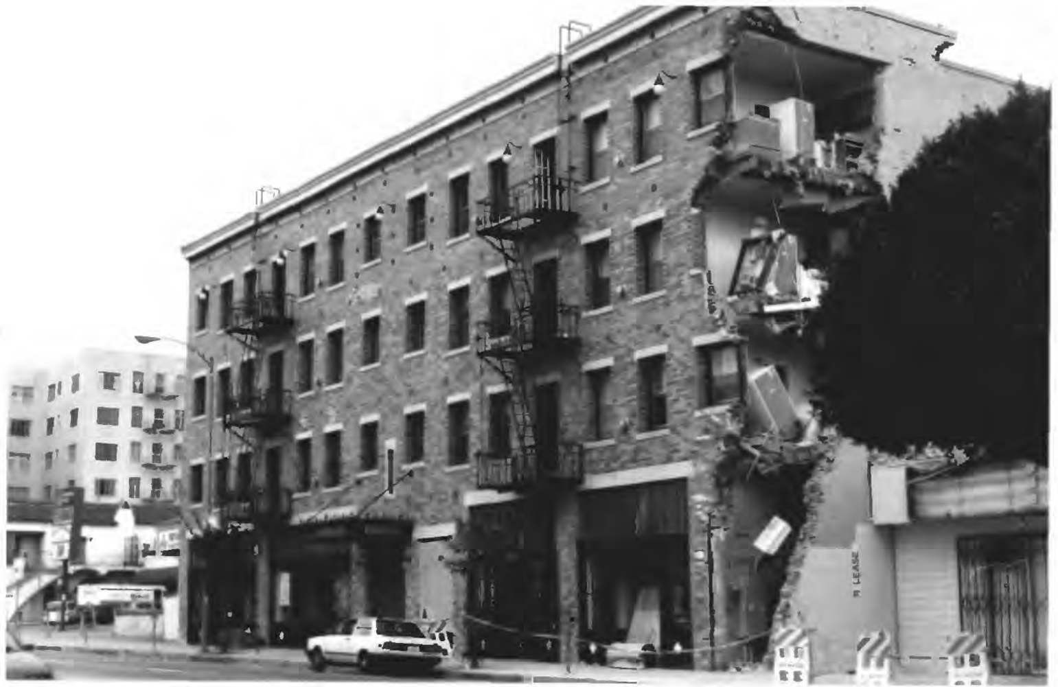
Figure 16. Damage to unreinforced masonry building, Hollywood Boulevard, Hollywood (listed under intensity VIII). At the time this picture was taken, most bricks and other debris on the sidewalk had been removed.
