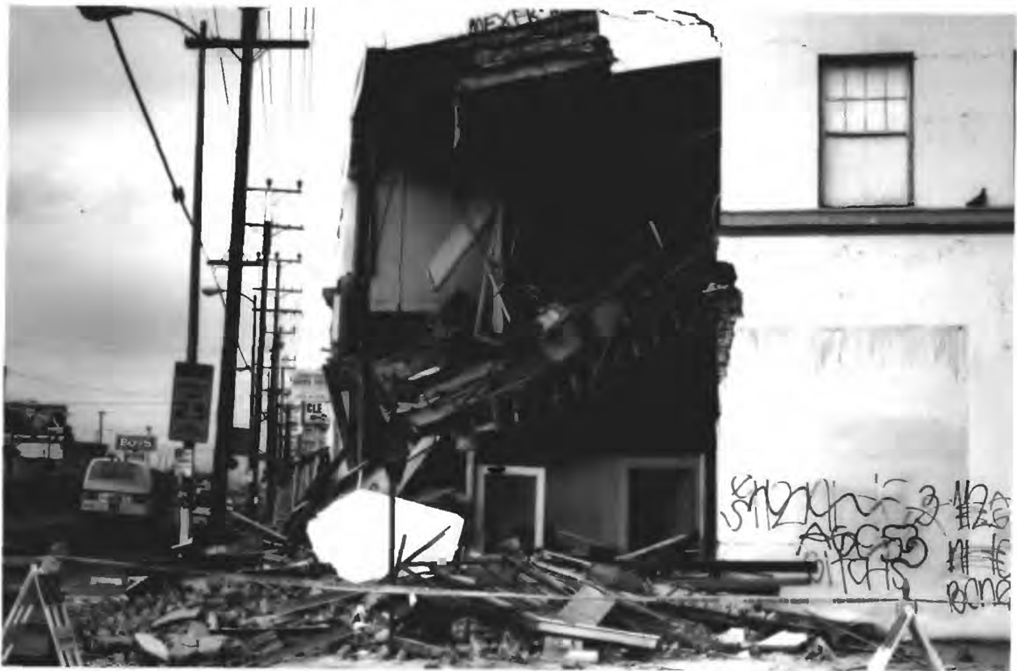
Figure 17. Damage to unreinforced masonry building, Los Angeles (West Adams) (listed under Intensity VIII).
