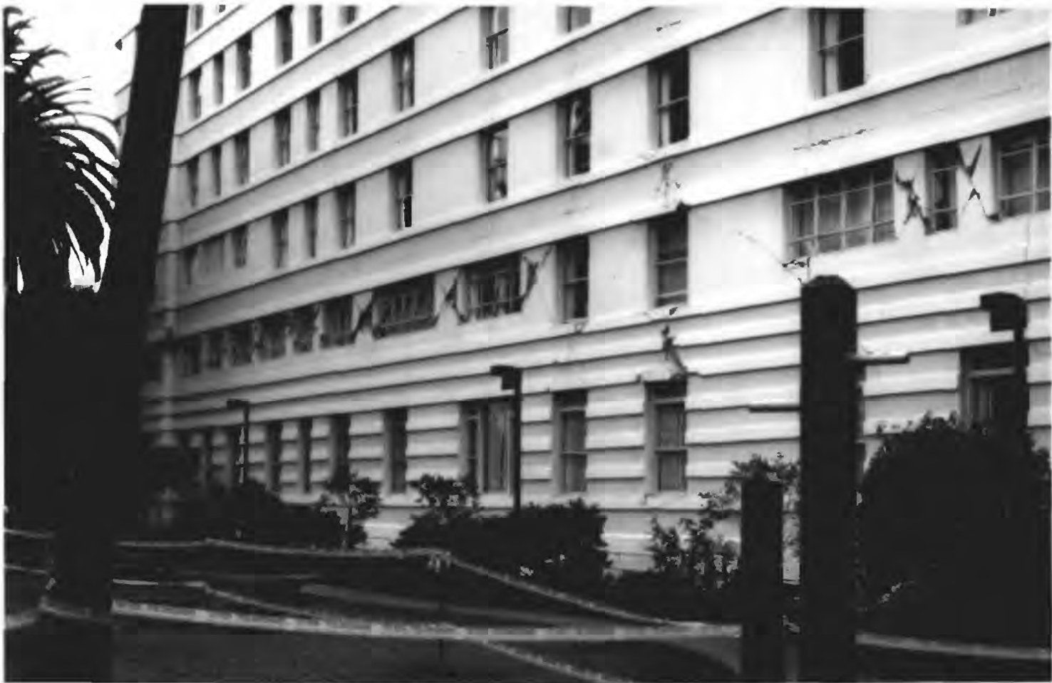
Figure 10. St. Johns Hospital, Santa Monica (this part of Santa Monica listed under intensity IX), showing diagonal shear cracks in piers at the second story level.
