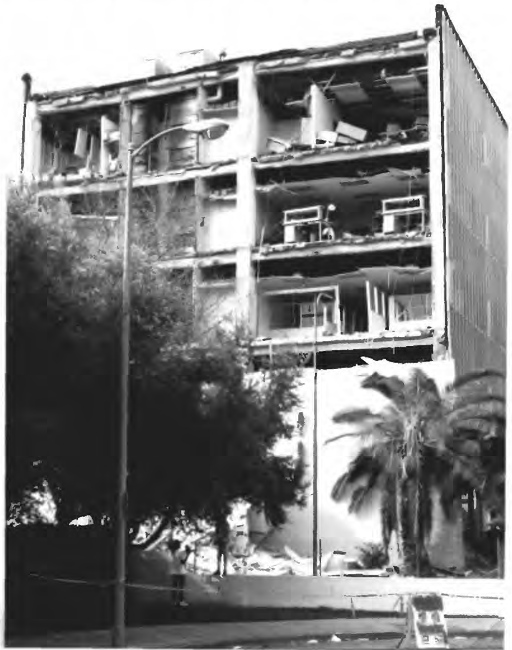
Figure 20. Office building with its interior exposed after cladding was shaken down, Reseda (listed under intensity VIII).
