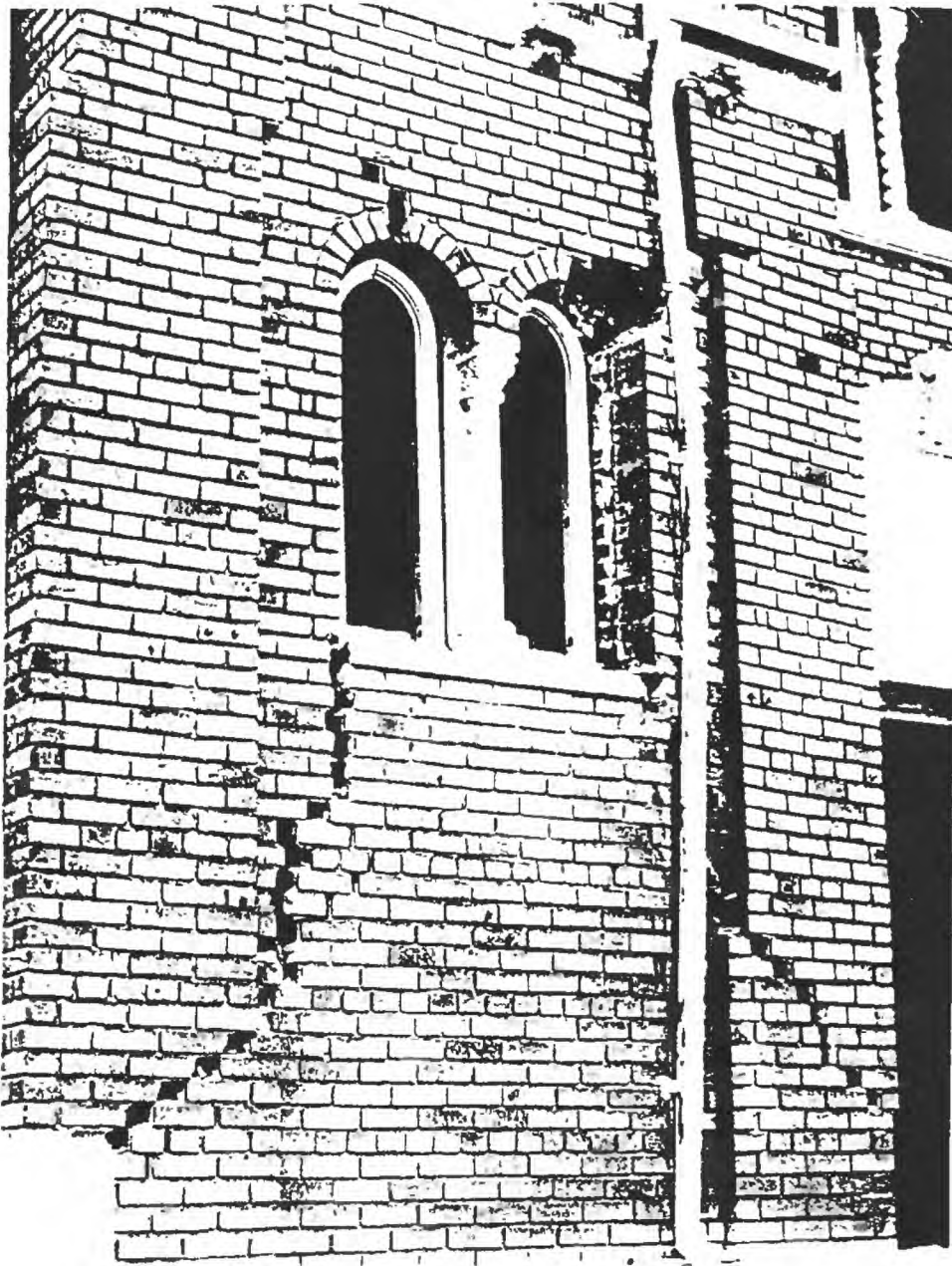
Figure 18. Damage to unreinforced masonry Southern Missionary Baptist church, Los Angeles (West Adams) (listed under Intensity VIII).
