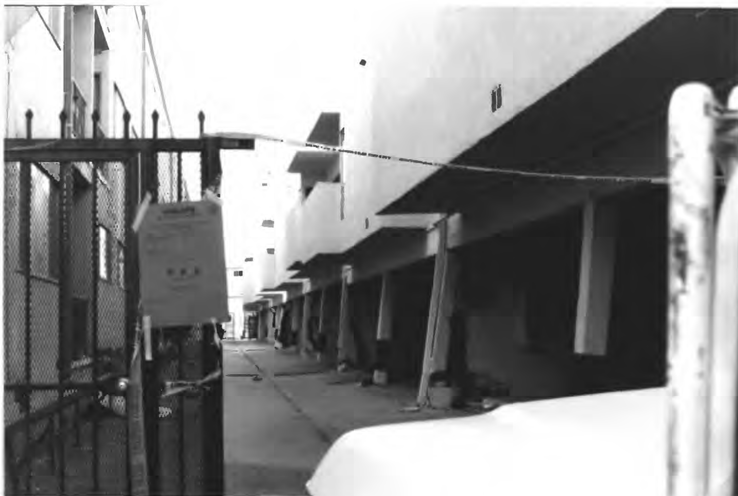
Figure 13. Displacement of upper stories of an apartment building over ground-floor parking area, Sherman Oaks (listed under intensity IX).
