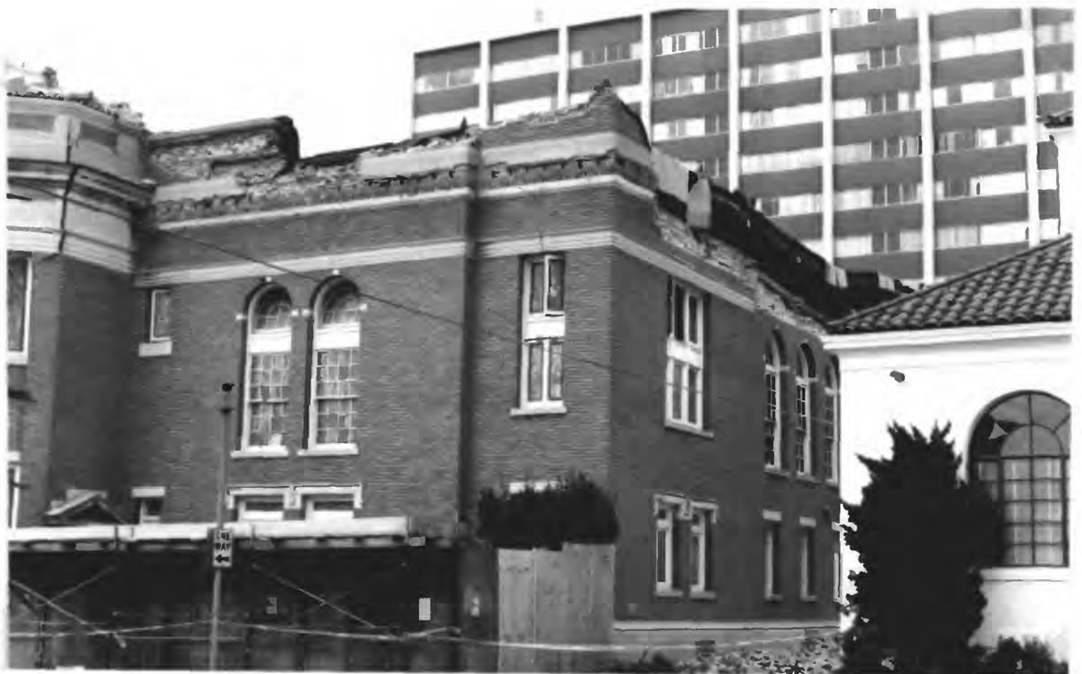
Figure 21. Damage to unreinforced masonry walls of the First Christian Church, Santa Monica (listed under intensity VIII).
