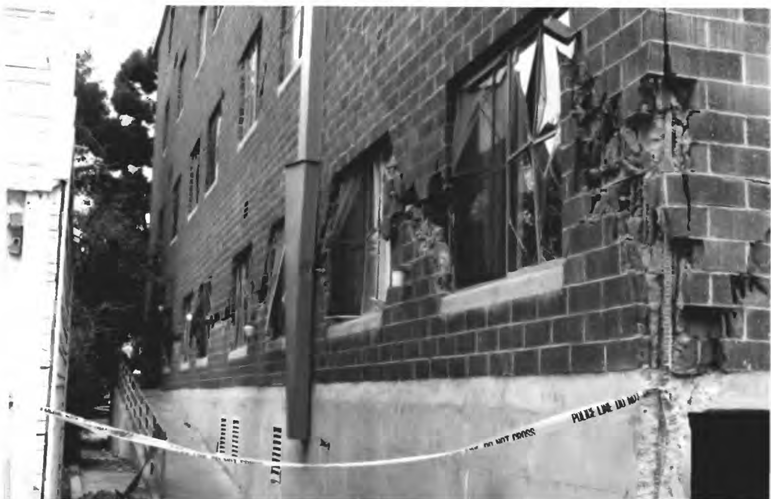
Figure 11. Damage to piers in the northwest-facing wall of the Berkeley East convalescent hospital, Santa Monica (this part of Santa Monica listed under intensity IX).
