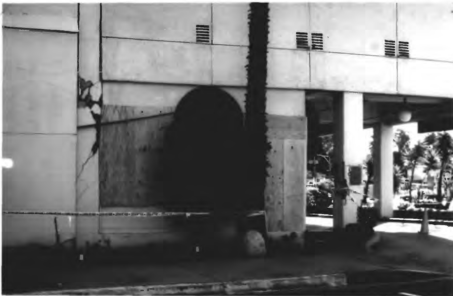
Figure 12. Damage to columns of the Radisson Hotel, Ventura Boulevard, Sherman Oaks (listed under intensity IX).
