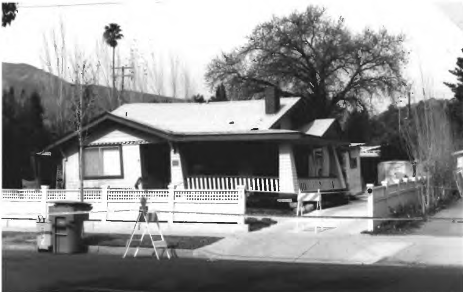
Figure 15. House shifted off its foundation, Fillmore (listed under intensity VIII).
