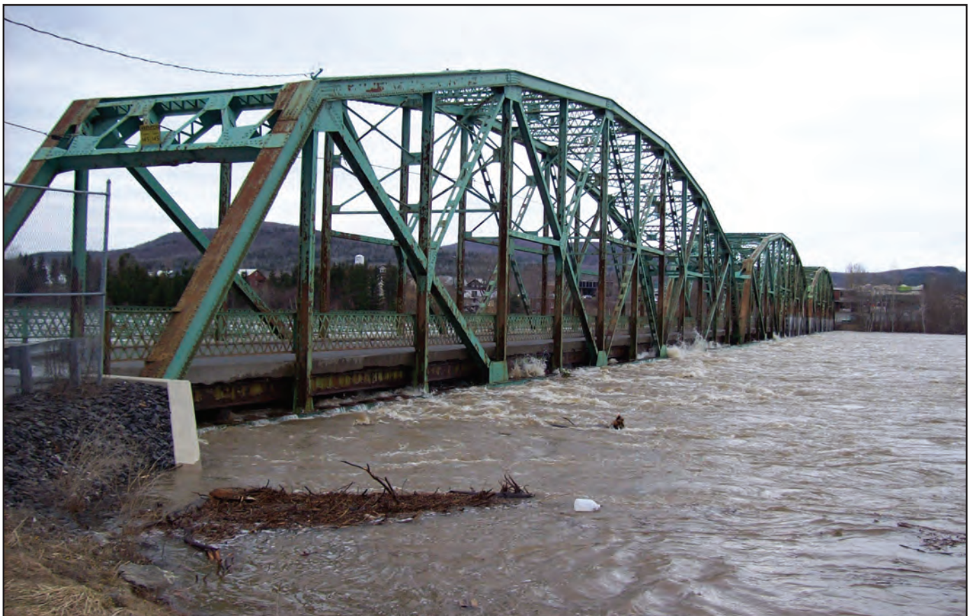
Figure 6. Flooding at International Bridge connecting Fort Kent, Maine, to New Brunswick, Canada, on April 30, 2008. (Photograph by Andrew Cloutier, U.S. Geological Survey)
